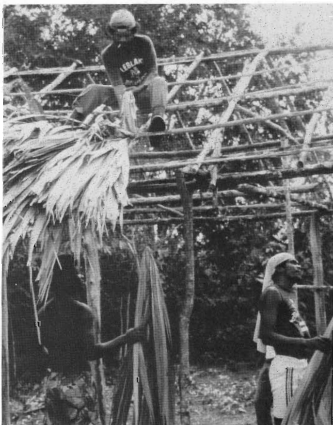
Fig. 5. Villagers of Bermudian Landing building a tourist shelter from local materials (photo by R. Horwich).
